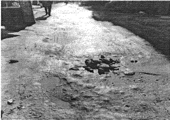
Condition of Roads in Ghitorni Village
